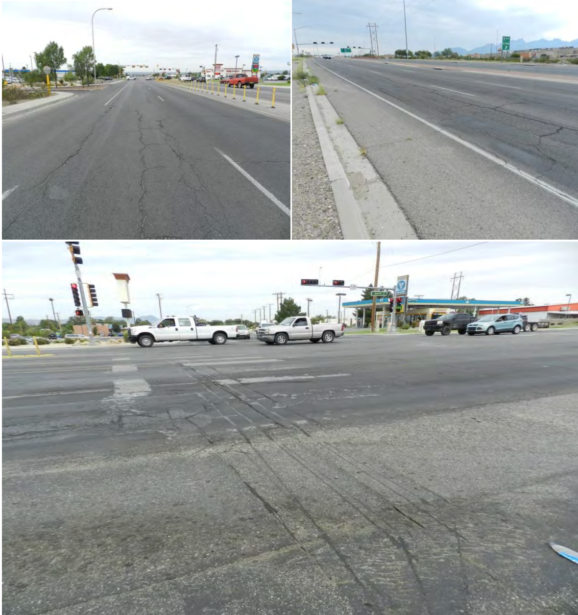
Figure 5: US 70 Pavement Conditions
